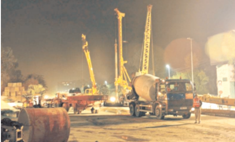
Work is yet to start again on Lahore's Signal Free Corridor by the LDA following the Supreme Court's suspension of the Lahore High Court's verdict 12
